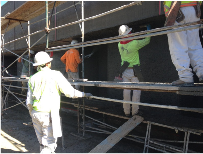
Date:02/10/16 Rutherford applying scratch coat of plaster at the exterior of the building.
