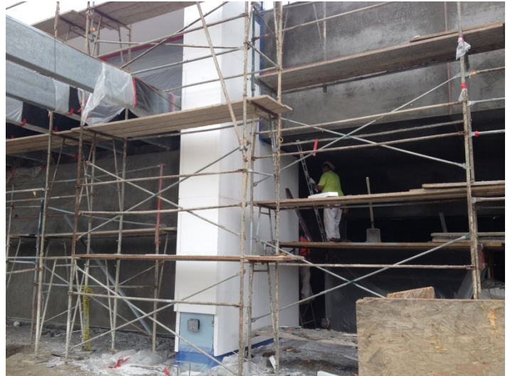
Date: 02/17/16 Rutherford detailing EIFS at East perimeter of the building, adjacent to book drop off.
