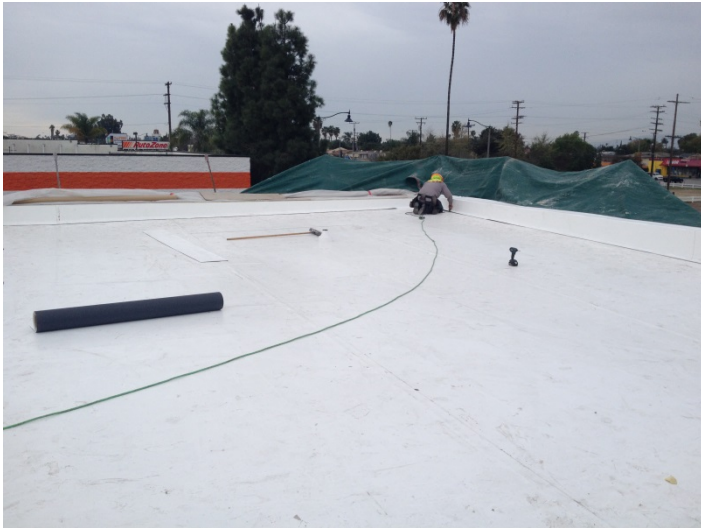
Date: 02/17/16 JP Witherow welding sarnafil membrane at parapet bases at South main roof elevation.
