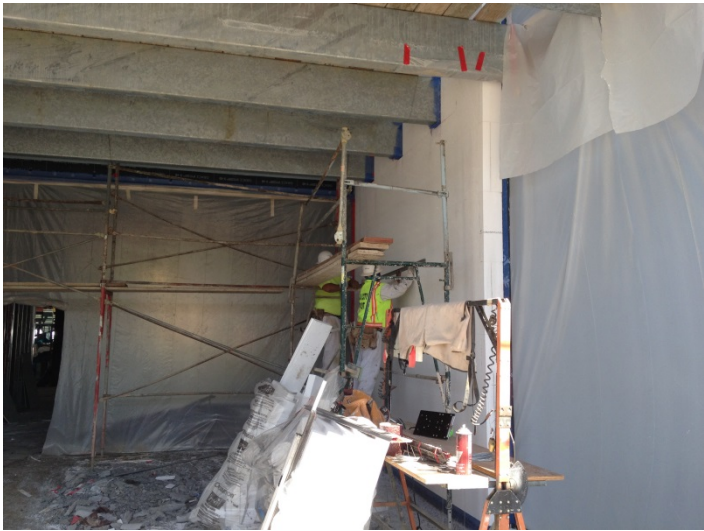
Date: 02/19/16 EIFS crew rasping and detailing EIFS at entrance to the Library.
