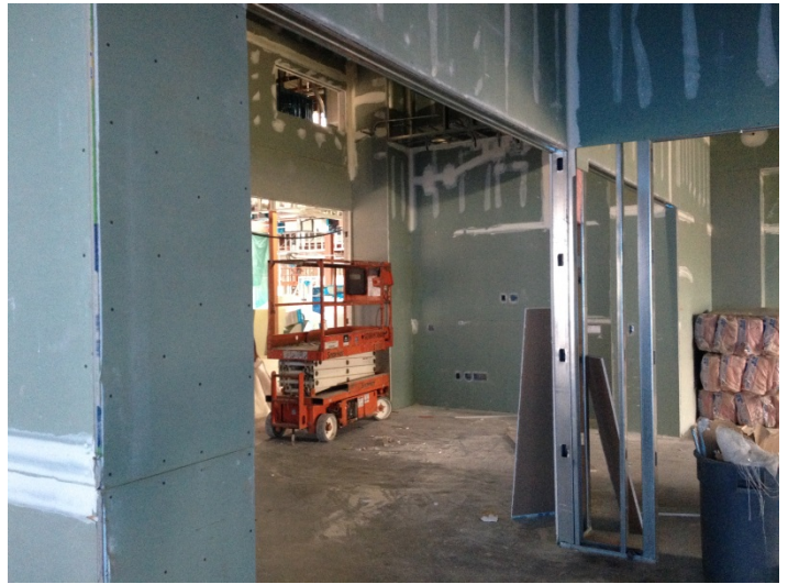
Date: 02/17/16 Progress of drywall installation at interior of the library. Conference room shown in picture above.
