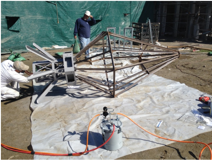
Date: 02/19/16 Painters priming tower spire in preparation for painting and hoisting onto structure.
