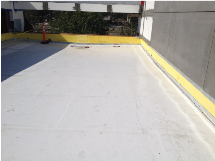
Date: 02/19/16 Previously installed flat bars at base of walls in courtyard area.
