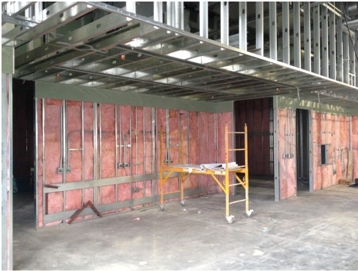
Date: 02/17/16 Progress of insulation work at interior walls, along main pathway entrance to the Library.
