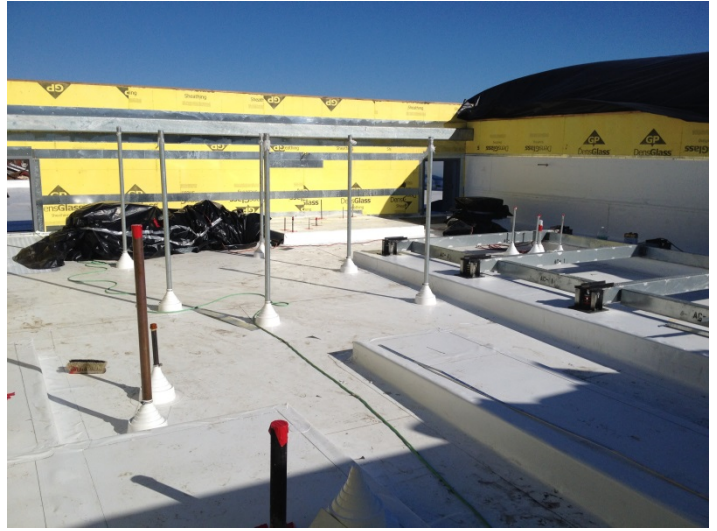
Date: 03/08/16 Progress of roofing installation at Mechanical Area I, above childrens collection area,
