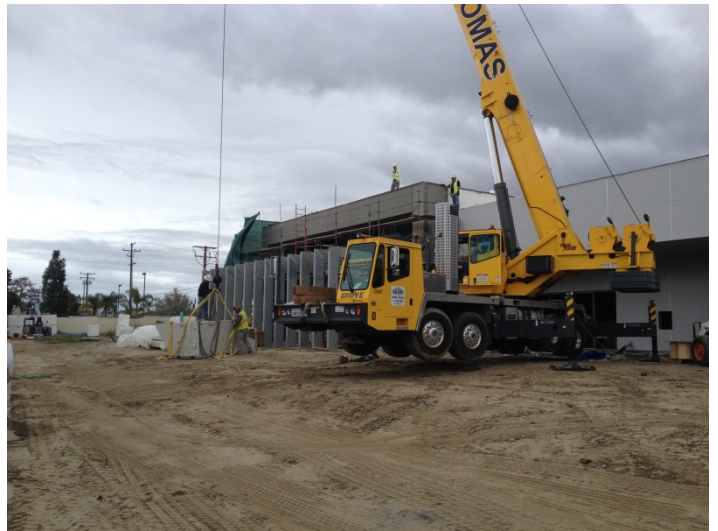
Date: 03/11/16 AC unit being prepped for lift and placement onto Mechanical Area II.
