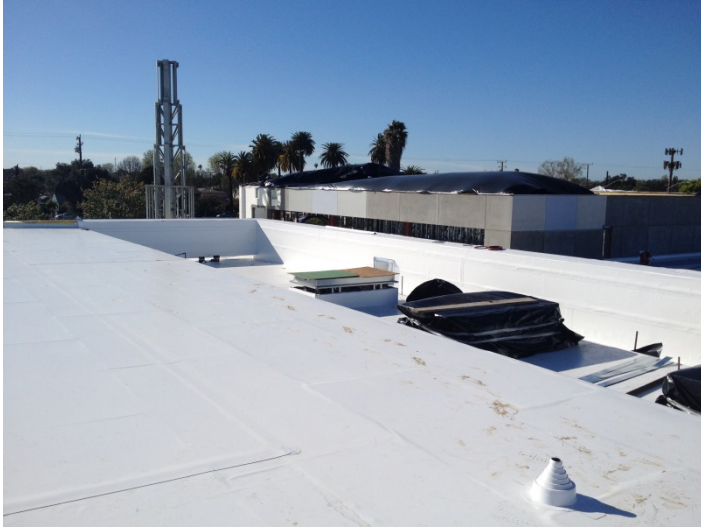
Date: 03/08/16 Progress of roofing installation at Mechanical Area I and above Community Rooms. Seams have been welded together and returned up the walls.
