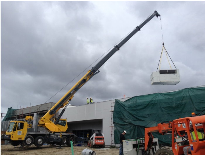
Date: 03/11/16 60 Ton AC unit being hoisted and lifted for placement onto roof.
