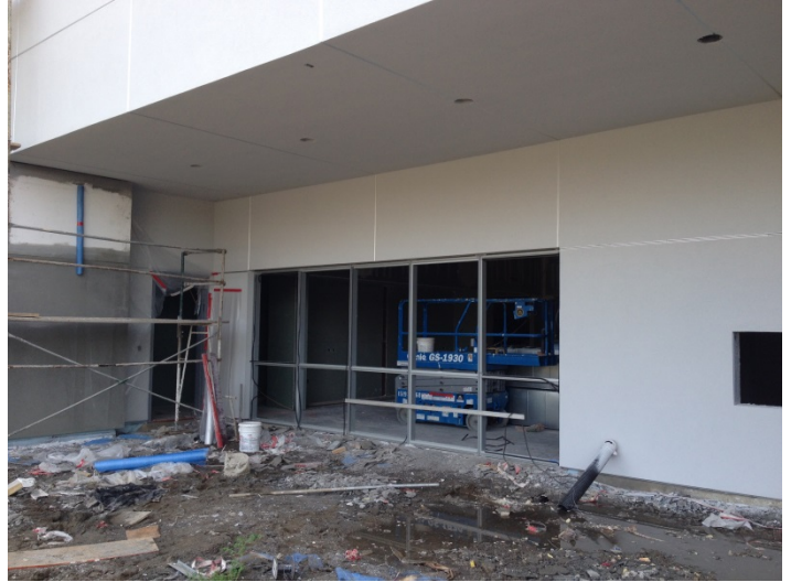
Date: 03/09/16 Curtain wall framing installation at classroom area, alongside East elevation adjacent to exterior book drop.
