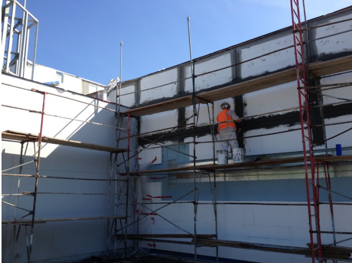
Date: 03/15/16 Rutherford detailing joints of EIFS at West elevation adjacent to tower.
