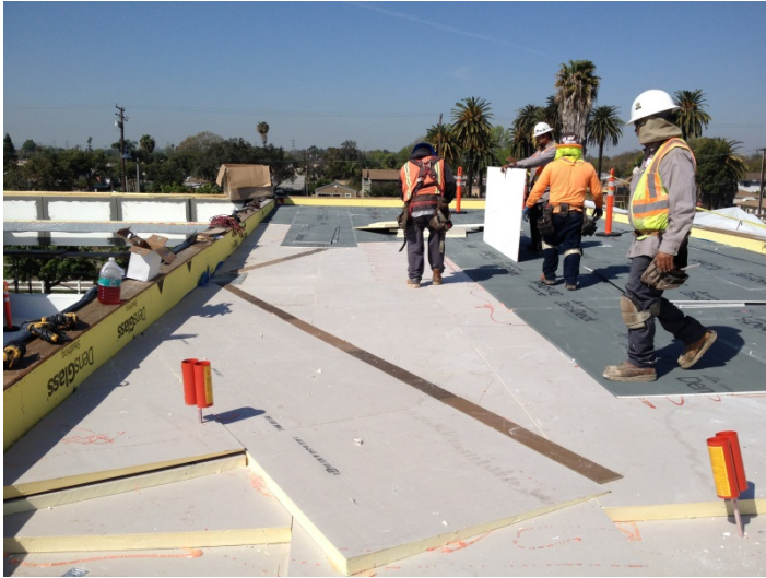
Date: 03/15/16 JP Witherow installing roofing at high elevation above the adult collection area.
