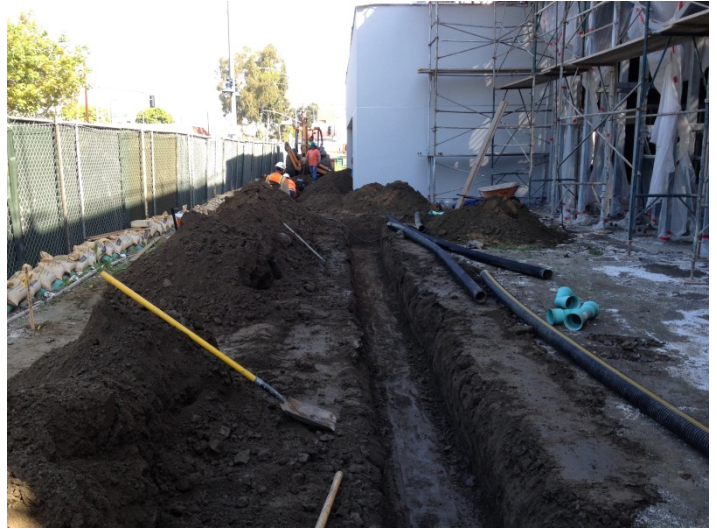
Date: 03/15/16 R. Brothers back onsite excavating for storm drain installation on West side of the building.
