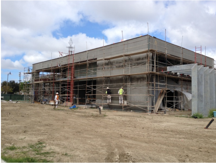
Date: 03/14/16 Rutherford applying genesis DM to face of EIFS panels along the South elevation.
