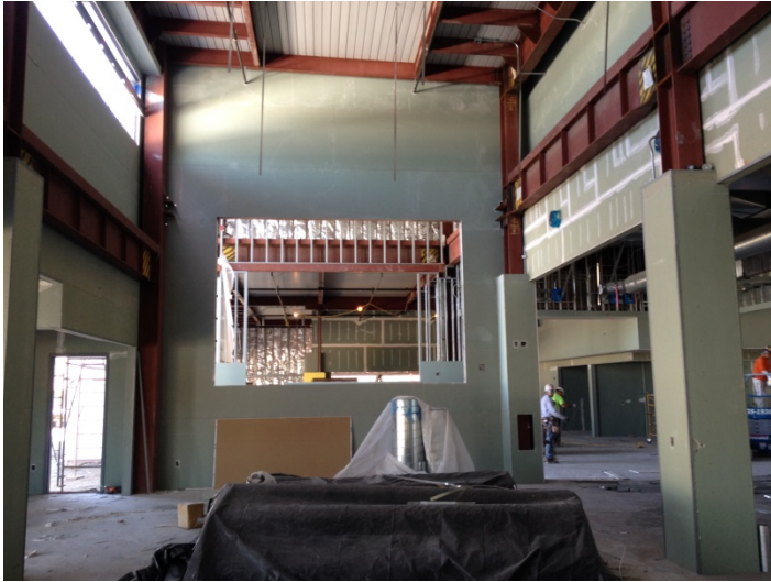
Date: 03/16/16 Progress of interior drywall installation, perspective from adult collection looking East to periodicals section.
