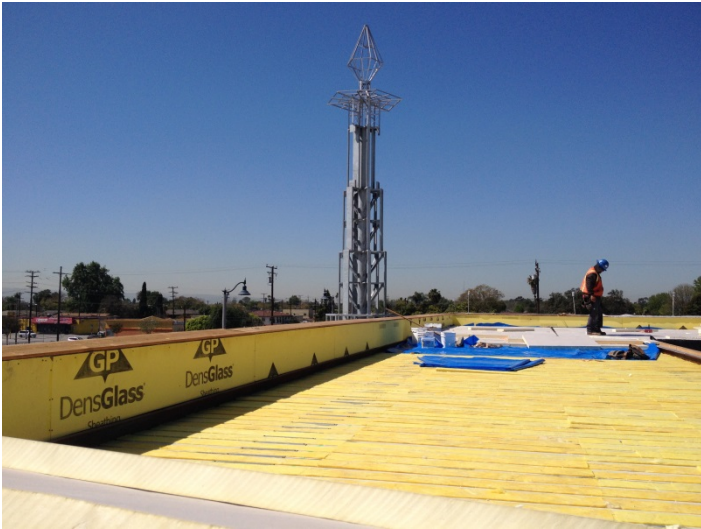
Date: 03/16/16 JP Witherow setting insulation and vapor barrier at high roof elevation, South of Mechanical I.
