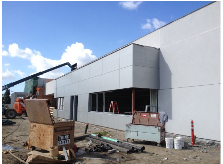
Date: 03/30/16 EIFS and Plaster finishes at the exterior of the library along the East elevation at the Family Learning Center.
