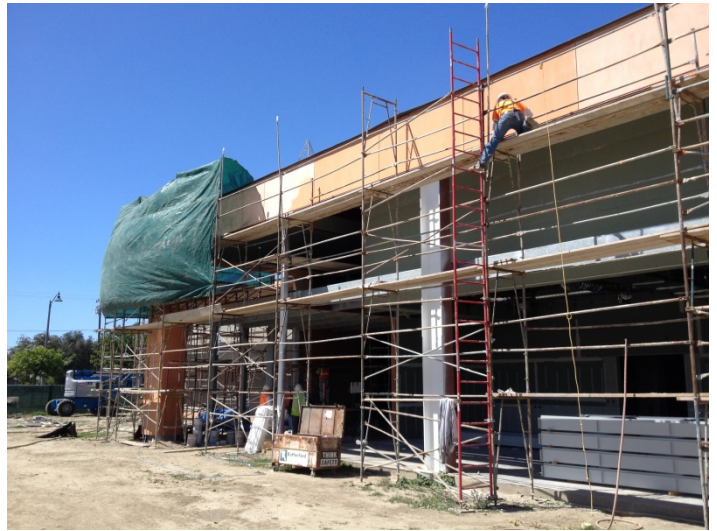
Date: 03/29/16 Dryvit continuing to sand / detail skim-it coat at South elevation of community room.
