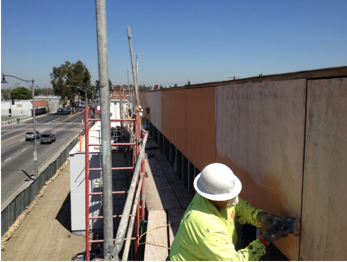
Date: 03/31/16 Rutherford continuing to sand / finish skim-it coat for EIFS along the West upper elevation.
