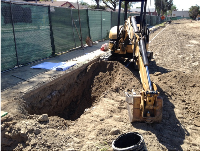
Date: 03/31/16 WCF beginning to excavate footings for site wall along Lime Avenue.
