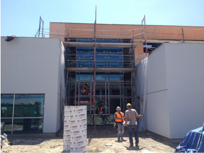
Date: 04/12/16 Glass being installed at curtain wall located at Periodicals Area at the North side of the building.
