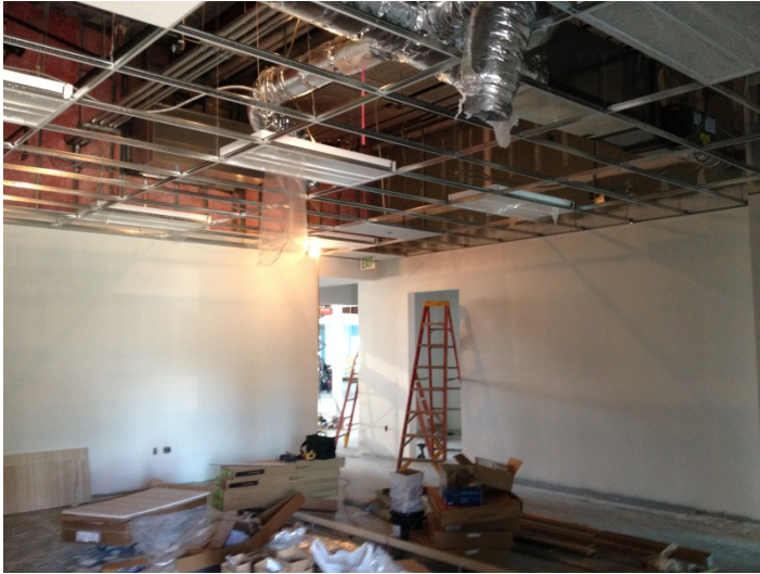
Date: 04/12/16 Light fixtures being dropped into place at ceiling grid in staff workroom area.
