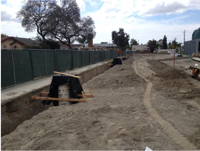
Date: 04/11/16 Formwork for light pole bases along East elevation of project site.
