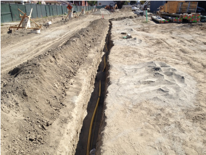
Date: 04/14/16 Gas line excavation along the East end of the project site.
