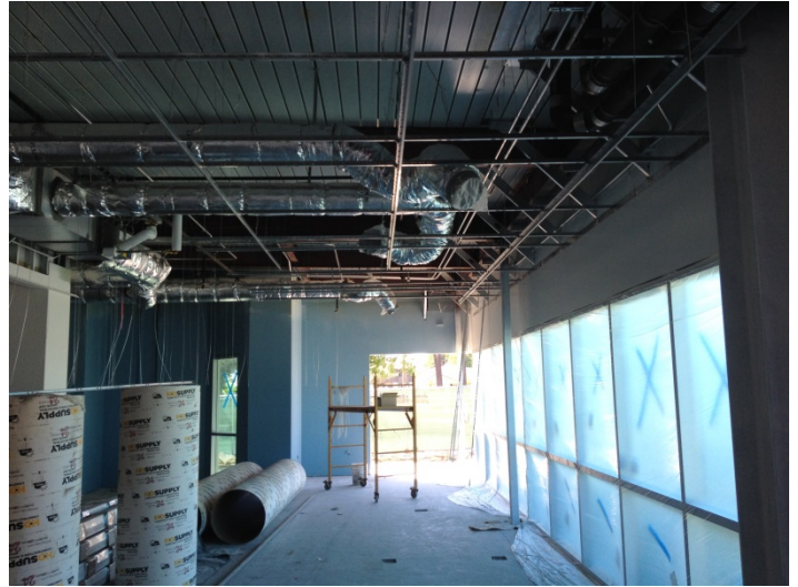
Date: 04/18/16 Progress of t-bar installation for metal ceiling at adult collection area.
