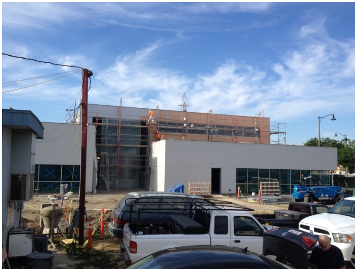
Date: 04/19/16 Rutherford applying primer to EIFS panels located at the upper North elevation of the building.
