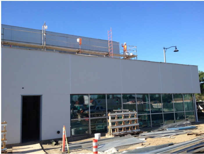
Date: 04/20/16 Rutherford applying final Reflect-it coat to EIFS panels on the upper North elevation.
