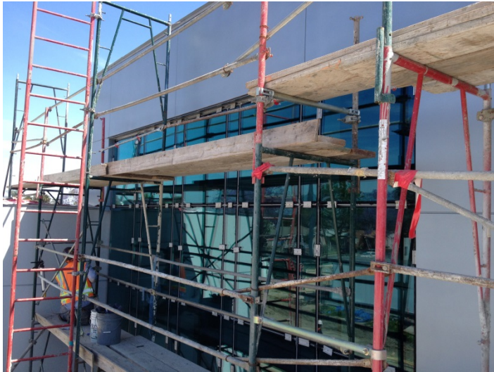
Date: 04/21/16 TMG caulking exterior joints at North curtain wall located at periodicals section.
