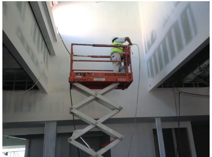
Date: 04/19/16 Quad County priming high ceiling walls in open space above children's collection.
