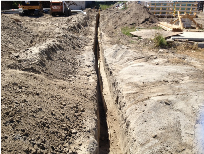
Date: 04/21/16 Gas line trench excavation and installation from retail space at the South end of the site.
