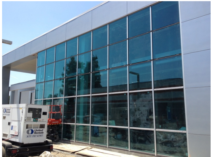
Date: 06/01/16 Installed vertical trim along the South elevation curtain wall at the large community room.
