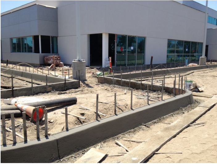
Date: 06/02/16 Curbs once formwork was removed at the Northeast corner of the site.
