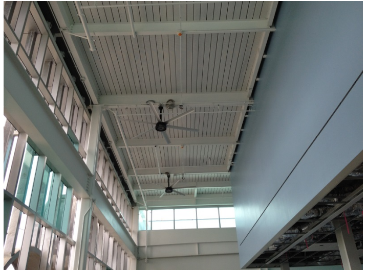
Date: 05/31/16 Installed ceiling fans above the West end of the children's collection space.
