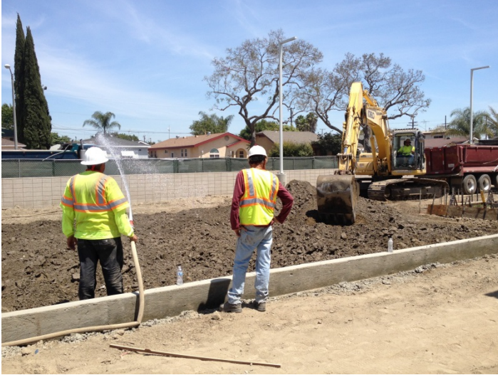
Date: 06/03/16 WCF continuing with site grading at the East end of the site.
