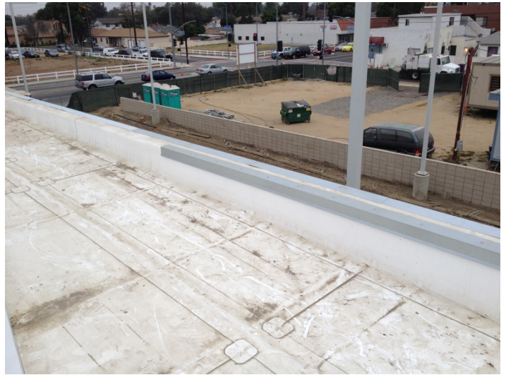
Date: 06/06/16 Metal cap flashing being installed at North main roof edge elevation.
