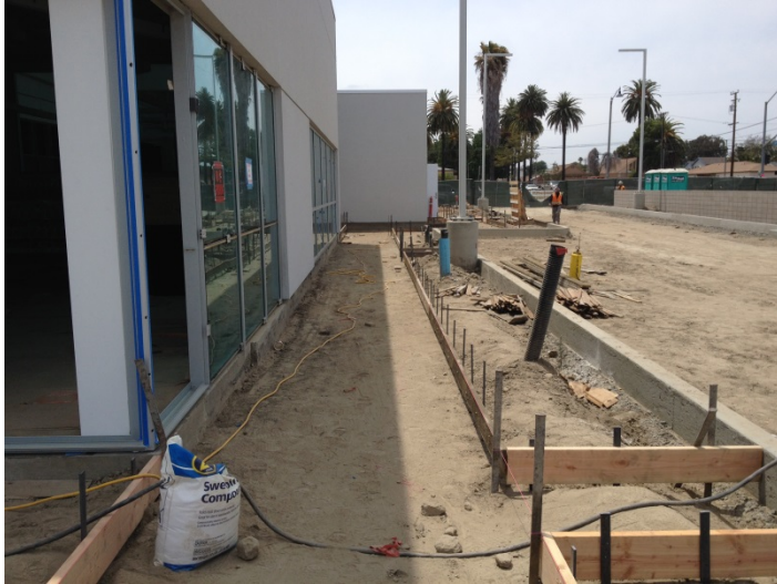
Date: 06/10/16 Constructed formwork for concrete paving at the North elevation of the building.
