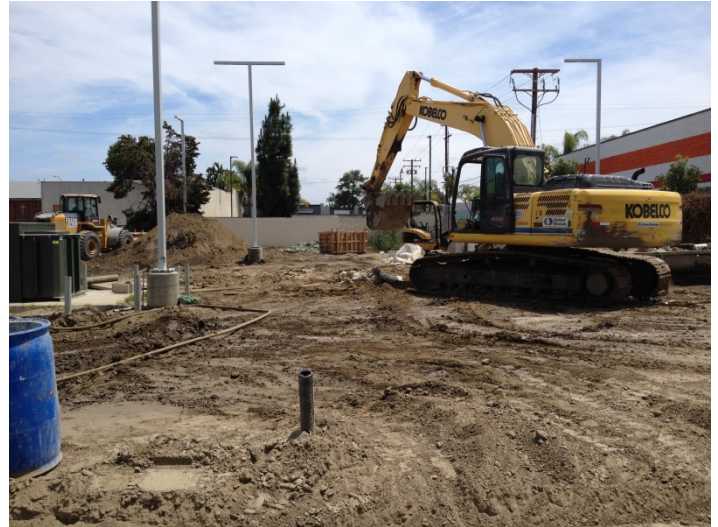
Date: 06/10/16 WCF continuing with grading at the South end of the site.
