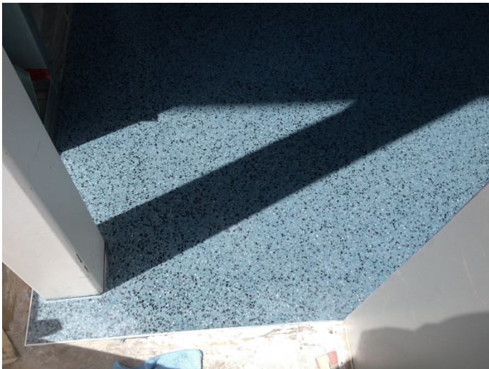
Date: 06/10/16 Finished terrazzo in the Southwest corner of the large meeting room.
