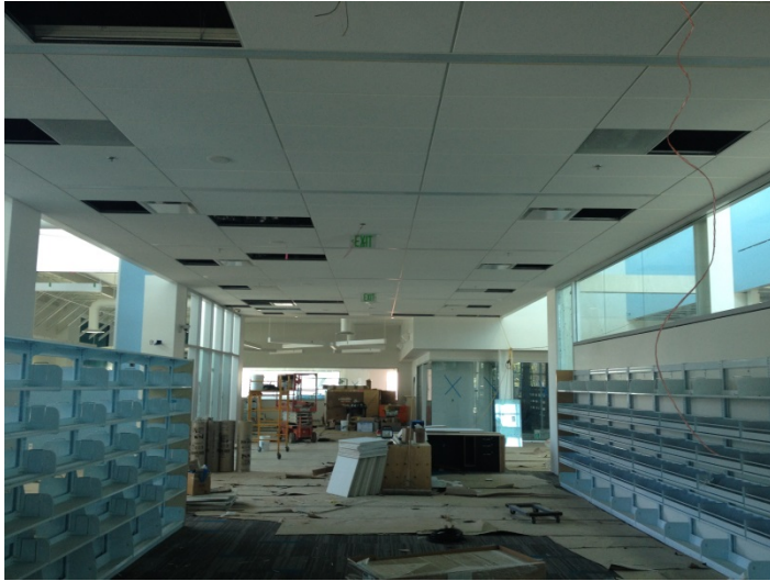
Date: 06/27/16 Installation of acoustic ceiling at adult collection leading to start of teen collection.
