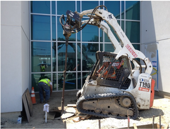
Date: 06/30/16 WCF excavating caisson for bubble wall at the North elevation of the building.
