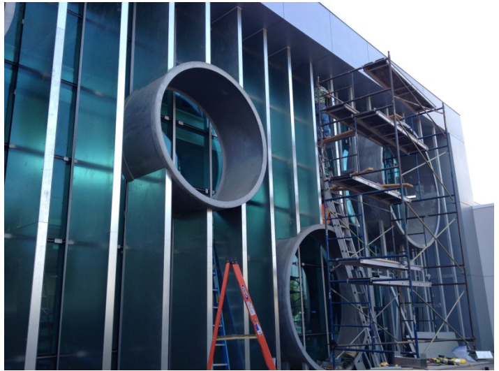
Date: 06/29/16 Valencia sheet metal continuing with installation of cladding at fin wall along West elevation.
