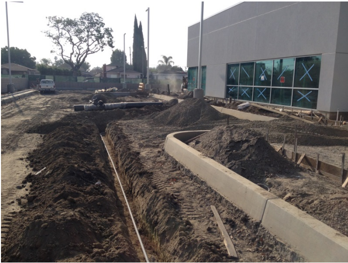
Date: 06/29/16 GBI trenching for installation of conduit to tie in light poles at the North end of the site.
