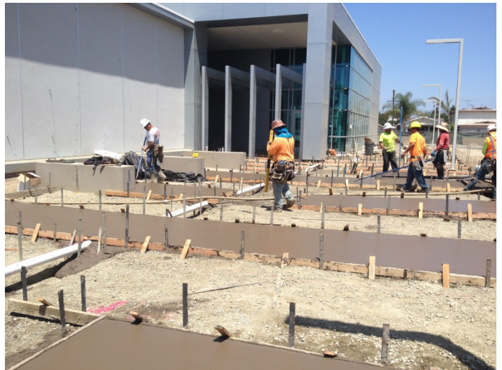
Date: 07/12/16 Concrete being placed at walkway to Library at the Southwest corner of the site.
