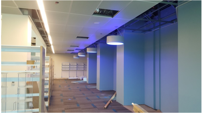
Date: 07/15/16 Lights fixtures installed and with power turned on in the adult collection area along the West elevation wall.
