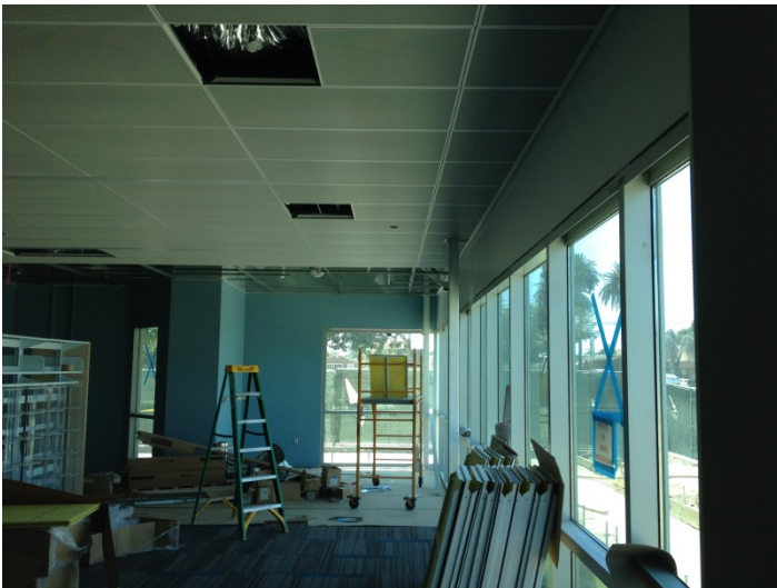
Date: 07/12/16 Progress of metal plank ceiling installation above the adult collection area.
