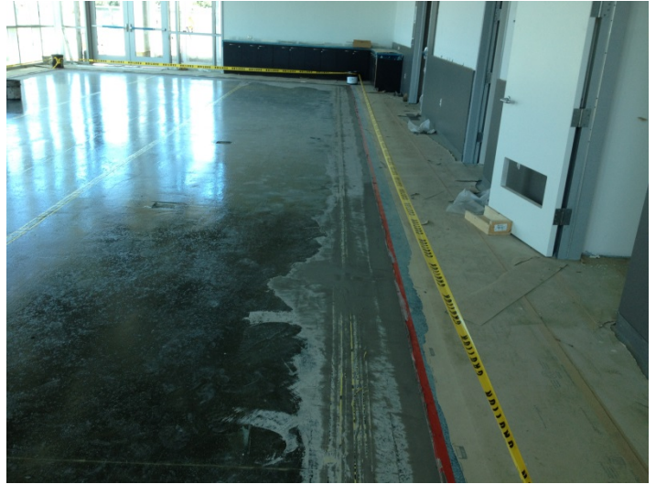
Date: 07/11/16 Large community room floor being prepped for installation of resilient flooring.
