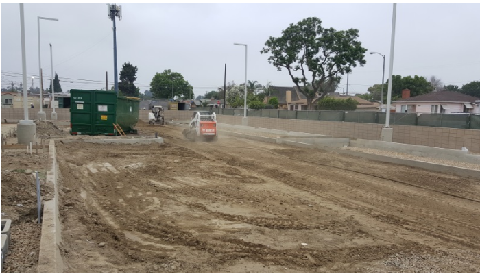
Date: 07/15/16 WCF performing additional grading at East elevation in preparation for asphalt paving.
