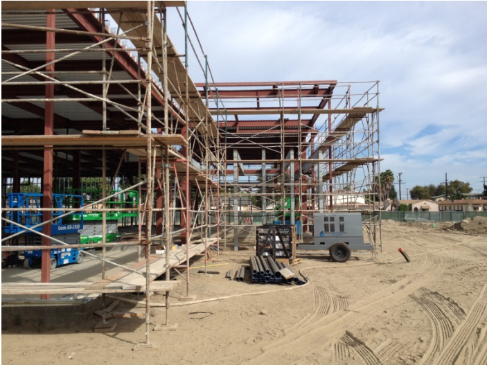
Date: 10/14/15 Rutherford continuing installation of scaffolding along the South perimeter of the building.
