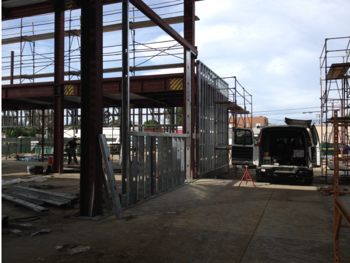
Date: 10/14/15 Rutherford installing interior metal stud in the periodical section of the library.
