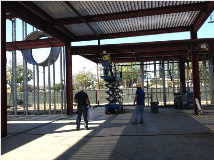
Date: 10/12/15 Fire Sprinkler subcontractor onsite to install sprinkler pipe throughout the building.
