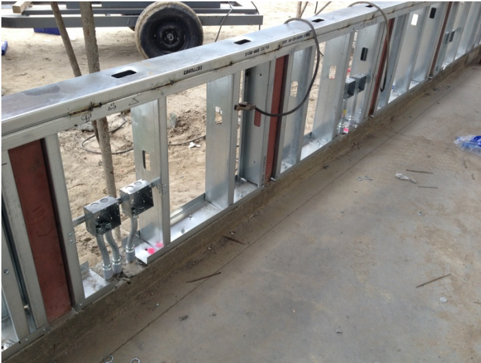
Date: 10/14/15 Electrician onsite to begin electrical rough in and install outlets along perimeter of the building.
