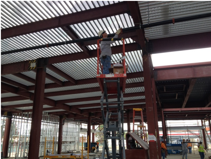
Date: 10/15/15 Red Fire continuing with installation of fire sprinkler pipe throughout the building.
