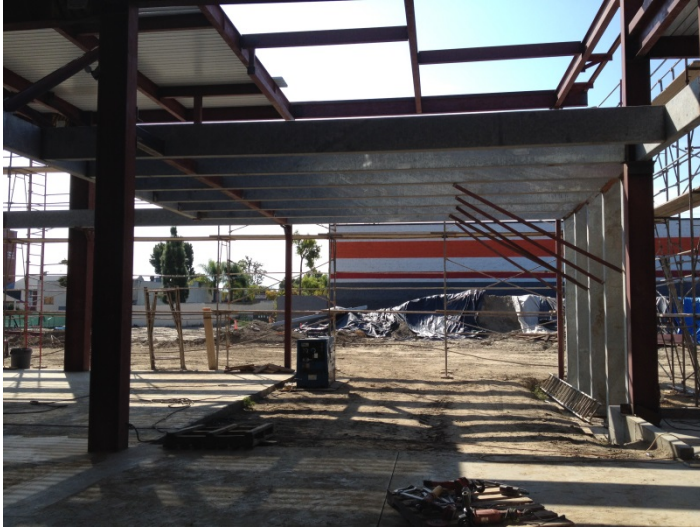
Date: 10/12/15 Trellis installed over entrance to Library at South end of the building.
